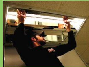
Retrofit Projects & Small Business
