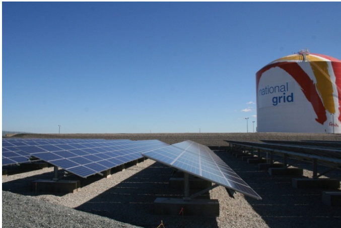
Photo: National Grid
