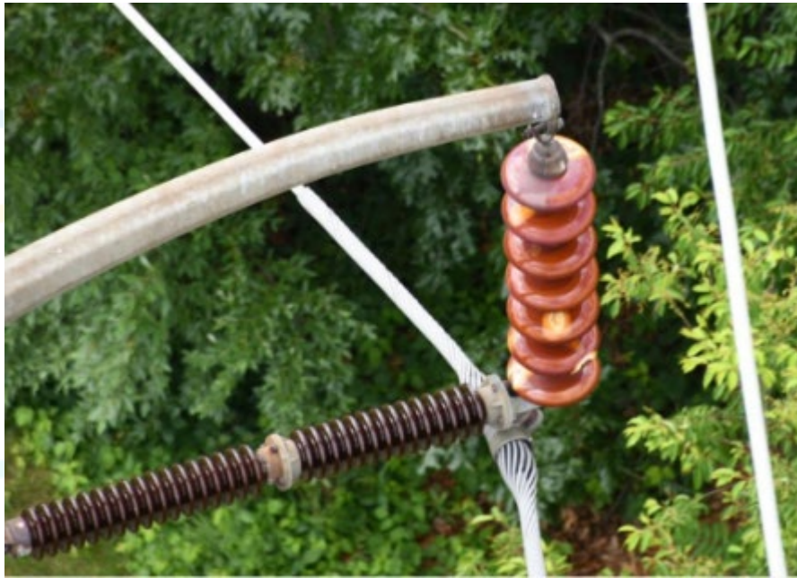
Flashed Insulator String with Insufficient Bell Count on E-183W Str 200
