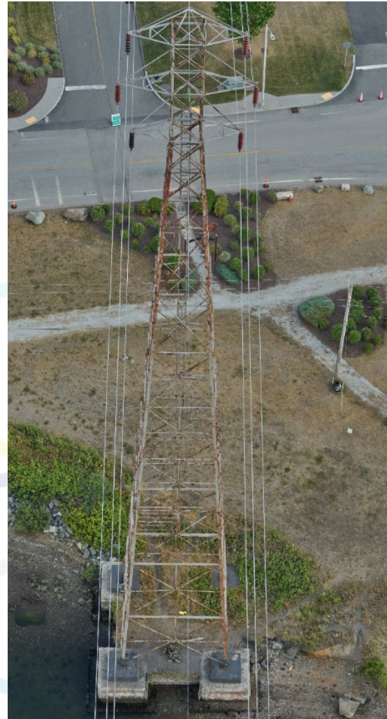
Severe Paint Chipping and Deterioration on E-183W Str 204
