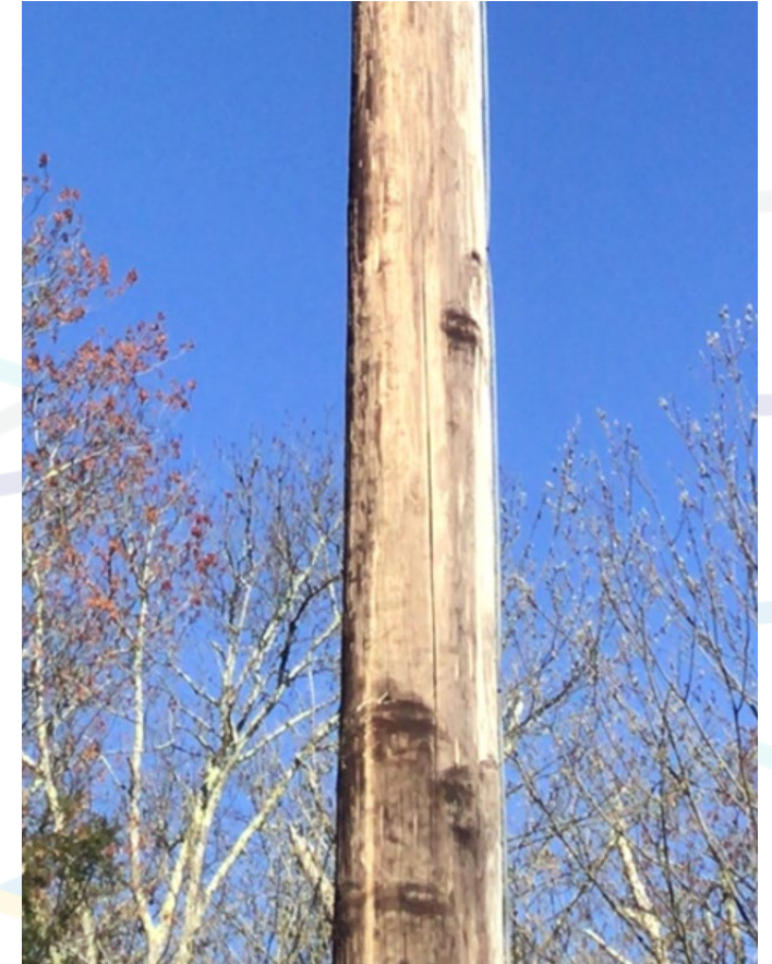
Structure Crack on L14 Str 19
