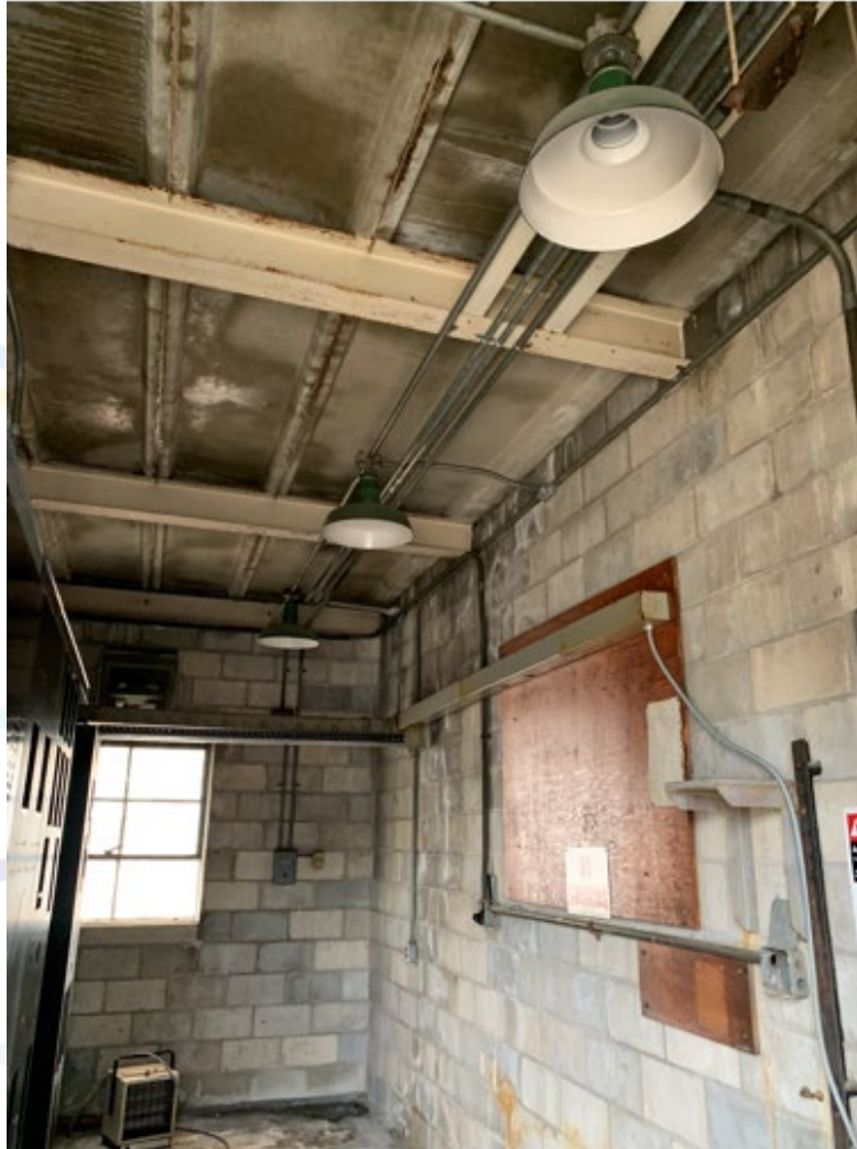
Canonicus Switchyard Building Interior
