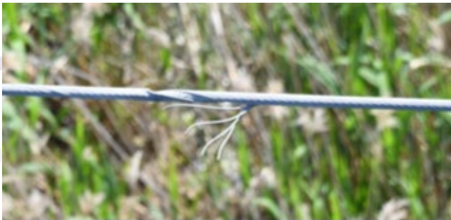
Broken Strands on M13 Span Between Str 82 and Str 83
