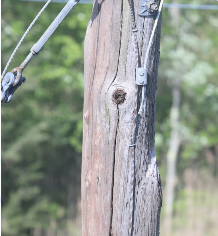
Pole Deterioration on T-172N Str 17
