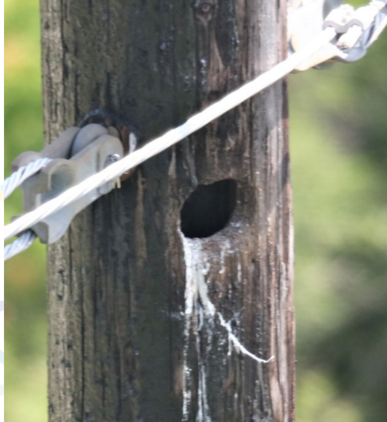
Woodpecker Damage on T-172N Str 126
