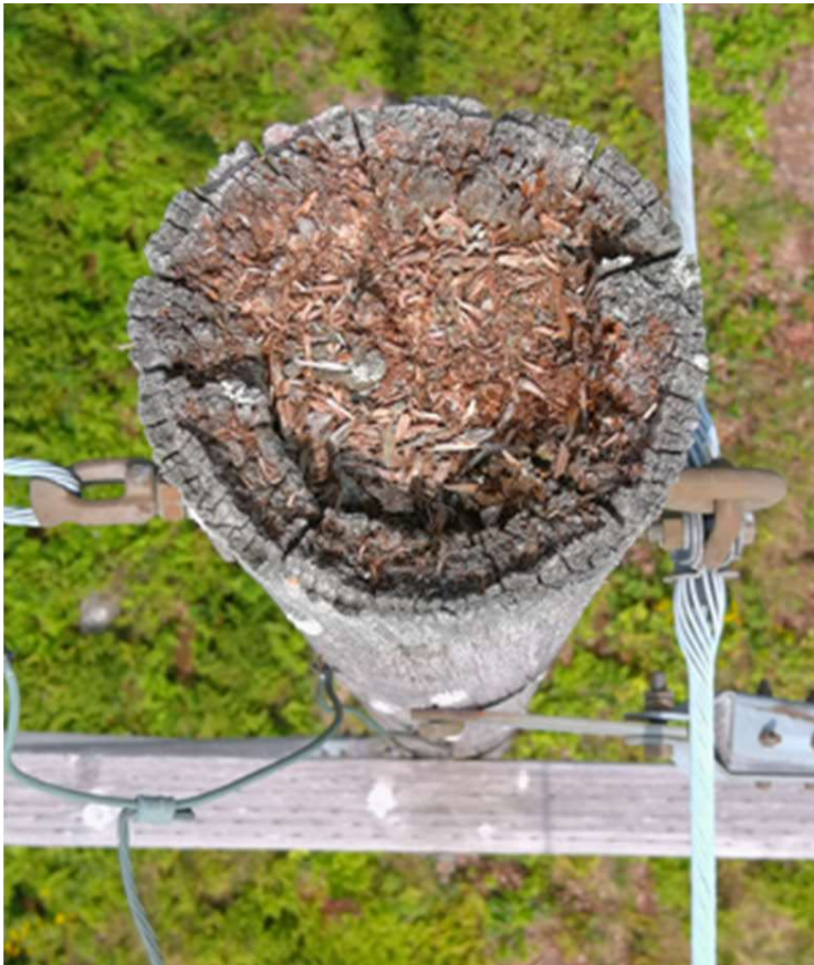
Structure 212 – Pole Top Rot & Rusted Hardware
