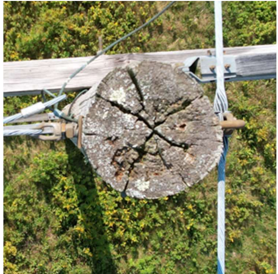
Structure 356 – Split Pole Top
