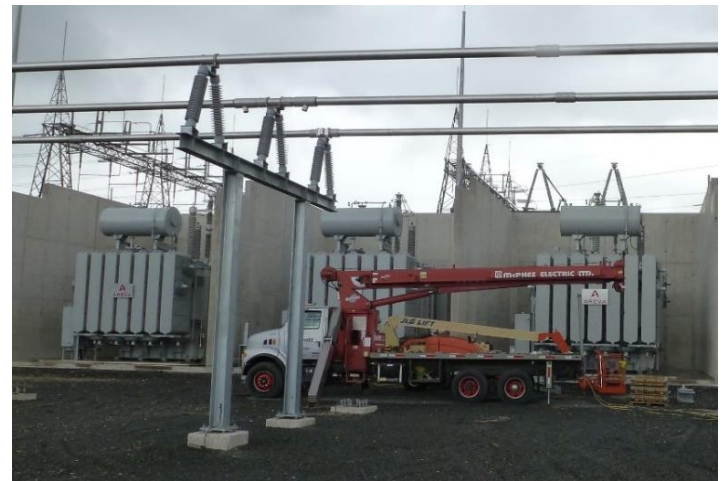
Photo illustrates the relative size of transformers on the New England bulk power system
