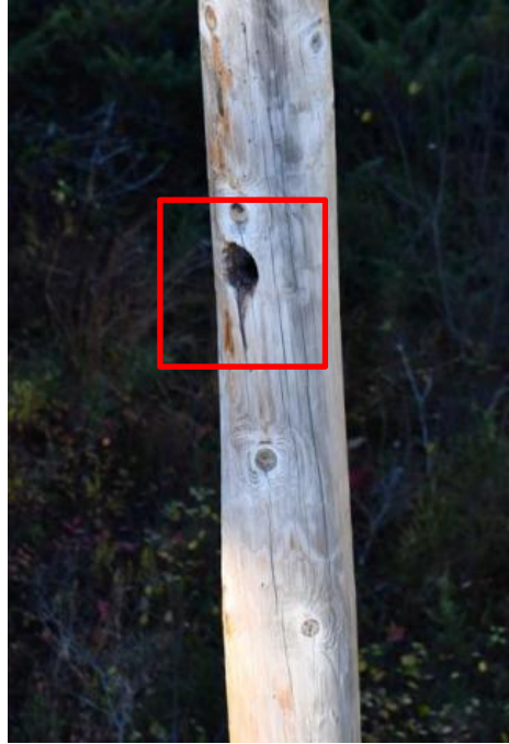
E-205E Str. 851 Installed 2009 Grade C – Woodpecker damage
