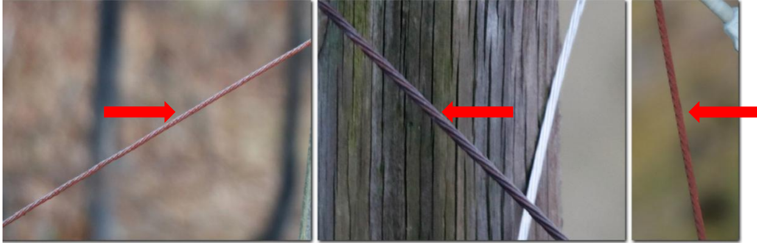
Entire circuit exhibiting deteriorated shieldwire condition due to corrosion
