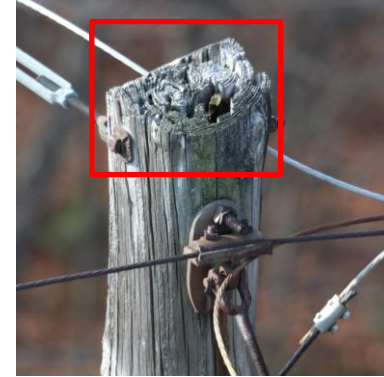
E-205W Str. 99 Installed 1962 Grade C – Pole top deterioration
