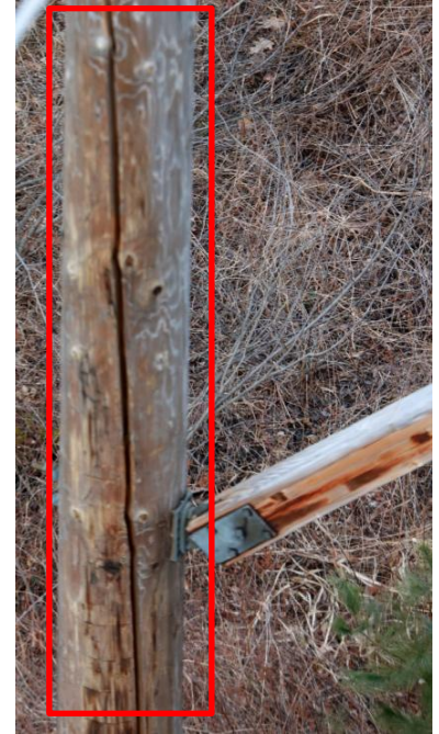
E-205E Str. 785 Installed 2009
