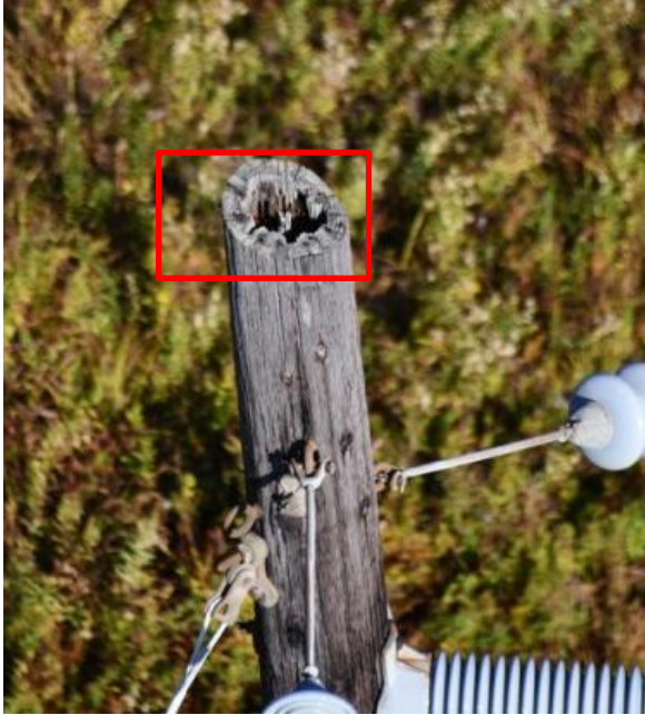
E-205E Str. 53 Installed 1972 Grade C – Pole top decay
