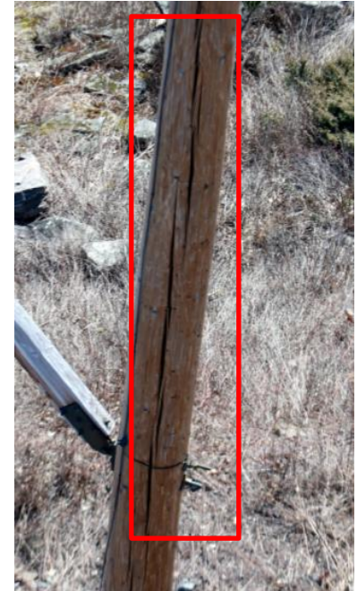
E-205E Str. 547 Installed 2009 Grade C – Deteriorated pole
