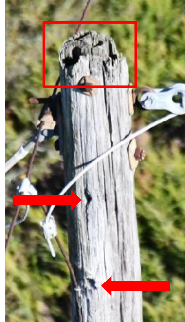
E-205E Str. 514 Installed 1962 Grade C – Pole top decay
