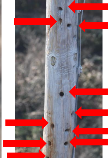
E-205W Str. 262 Installed 2000 Grade C – Woodpecker damage
