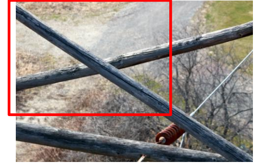
E-205E Str. 471 Installed 1962 Grade C – Deteriorated pole
