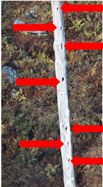
E-205W Str. 135 Installed 1962 Grade C – Woodpecker damage
