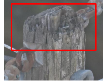
E-205W Str. 225 Installed 1962 Grade C – Pole top deterioration
