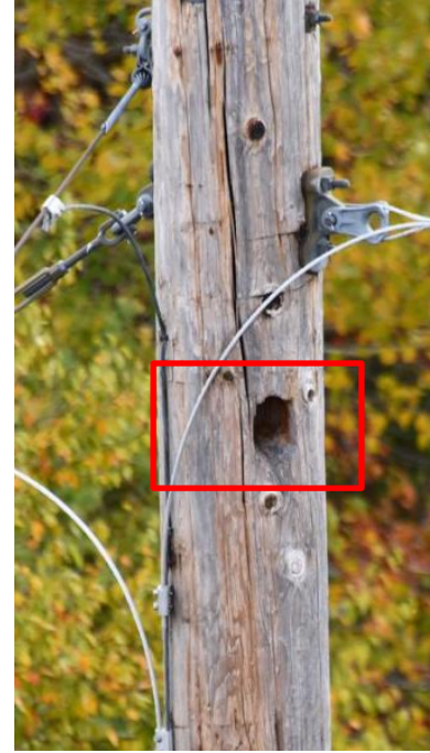
E-205E Str. 776 Installed 2009 Grade C – Woodpecker damage
