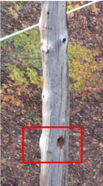
E-205W Str. 160 Installed 1962 Grade C – Woodpecker damage
