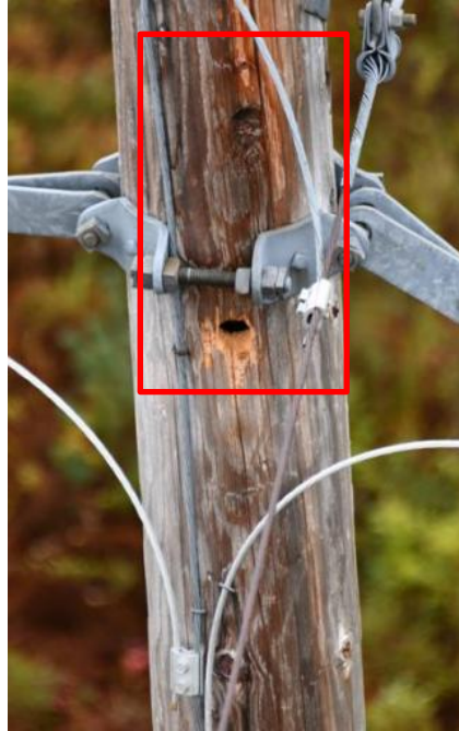
E-205E Str. 711 Installed 1995
