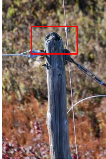
E-205E Str. 280 Installed 1962 Grade C – Pole top decay
