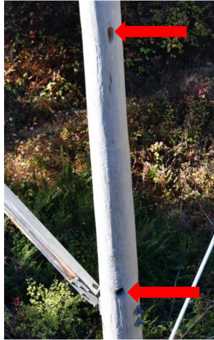
E-205E Str. 917 Installed 2010
