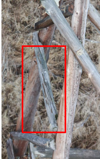
E-205E Str. 423 Installed 1962 Grade C – Deteriorated pole
