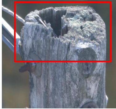
E-205W Str. 215 Installed 1962 Grade C – Pole top deterioration
