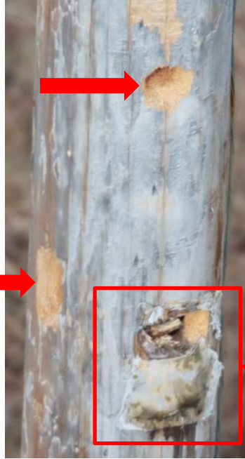
E-205E Str. 676 Installed 2009 Grade C – Woodpecker damage
