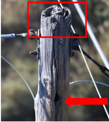
E-205W Str. 12 Installed 1962 Grade C – Pole top deterioration
