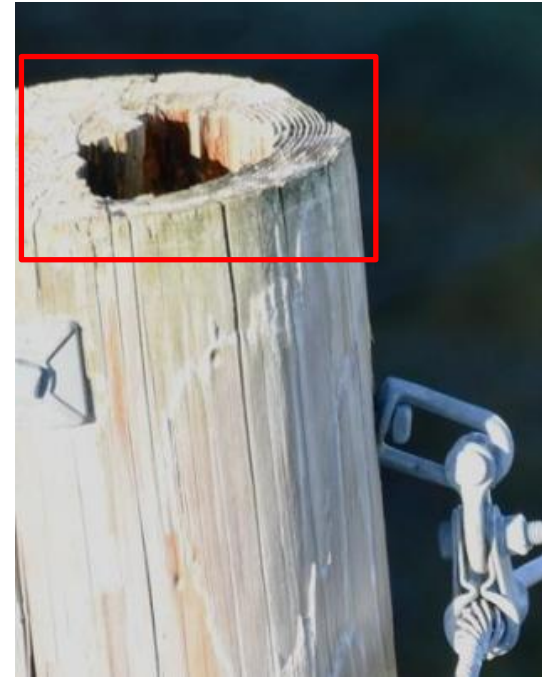
E-205E Str. 868 Installed 2009 Grade C – Deteriorated pole top
