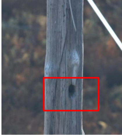
E-205W Str. 203 Installed 1981 Grade C – Woodpecker damage
