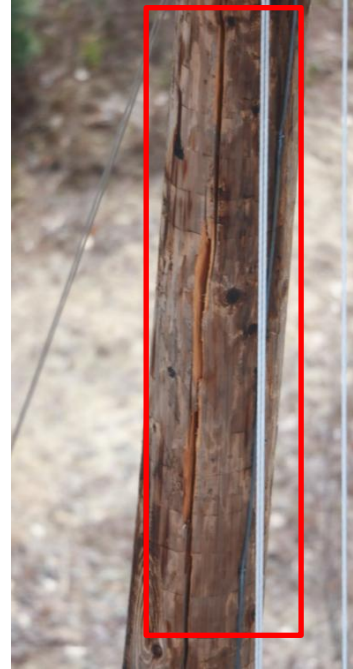
E-205E Str. 739 Installed 2009
