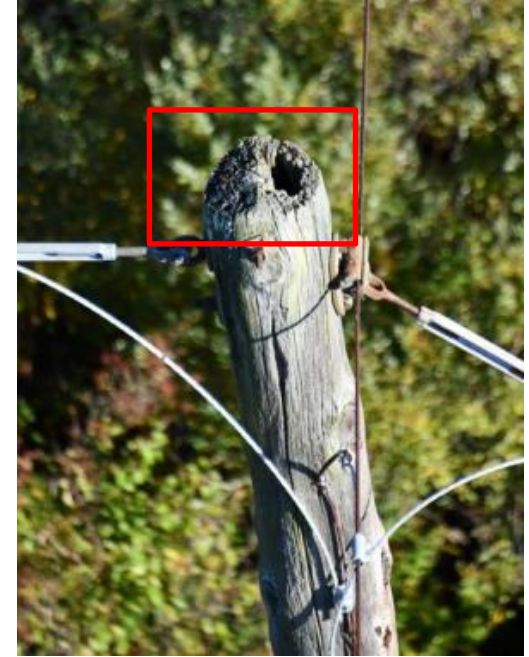
E-205E Str. 283 Installed 1962 Grade C – Pole top decay
