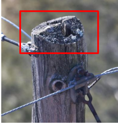
E-205W Str. 21 Installed 1962 Grade C – Woodpecker damage
