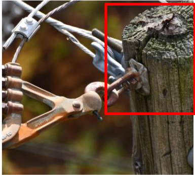
E-205W Str. 167 Installed 1962 Grade C – Pole top deterioration
