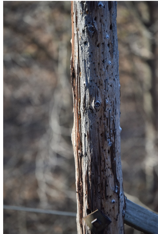
K22 Line Severely Weathered Pole
