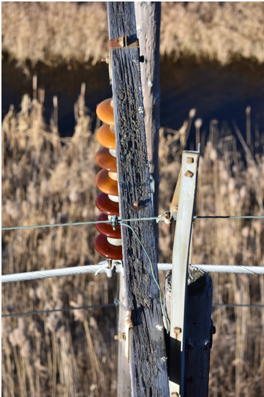
K22 Line Rotten Crossarm
