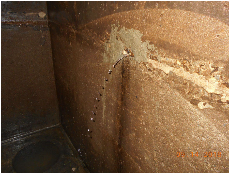
Line 1722 – Vault 5671 Active Water Leak
