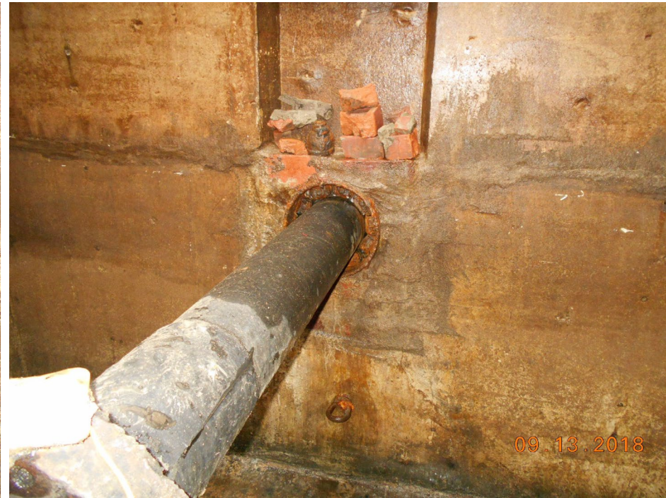
Line 1704 – Vault 5660B North Duct Showing Signs of Efflorescence
