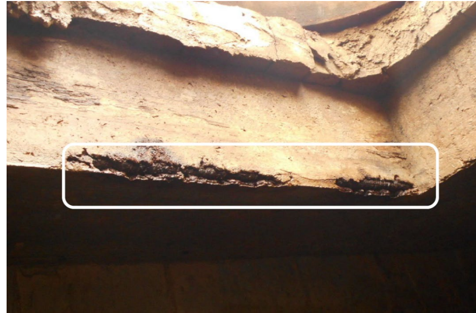
Line 1704 – Vault 5660A Exposed Rebar and Rust in Vault Ceiling
