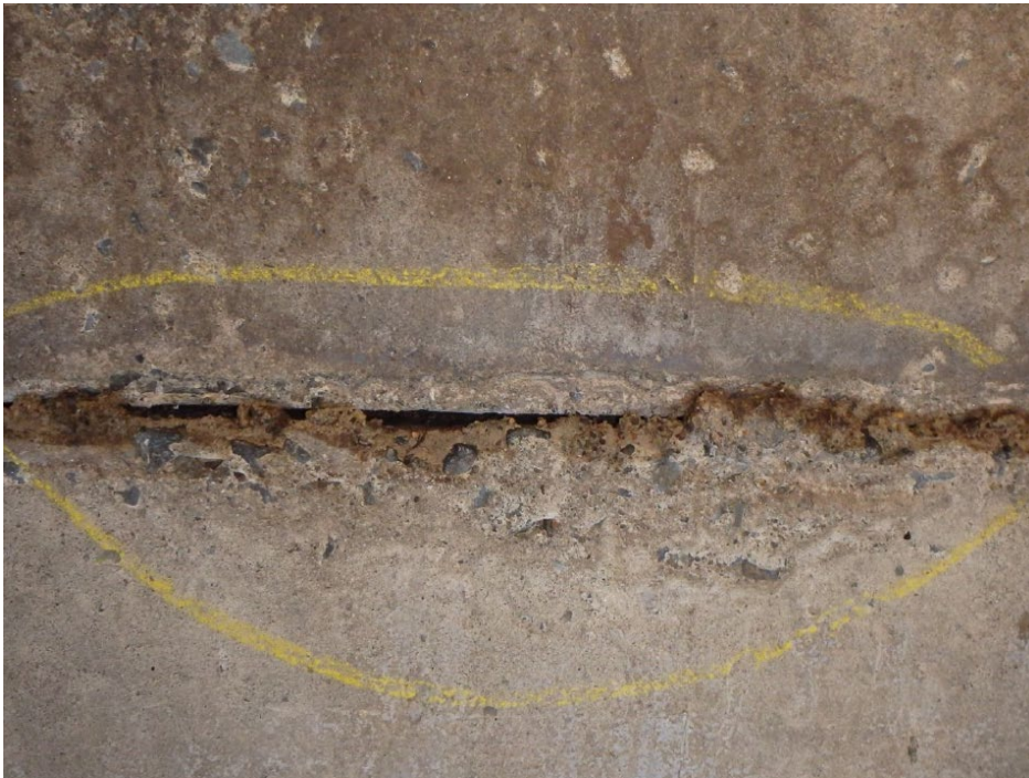
Line 1722 – Vault 5667A Deep Spall in Wall
