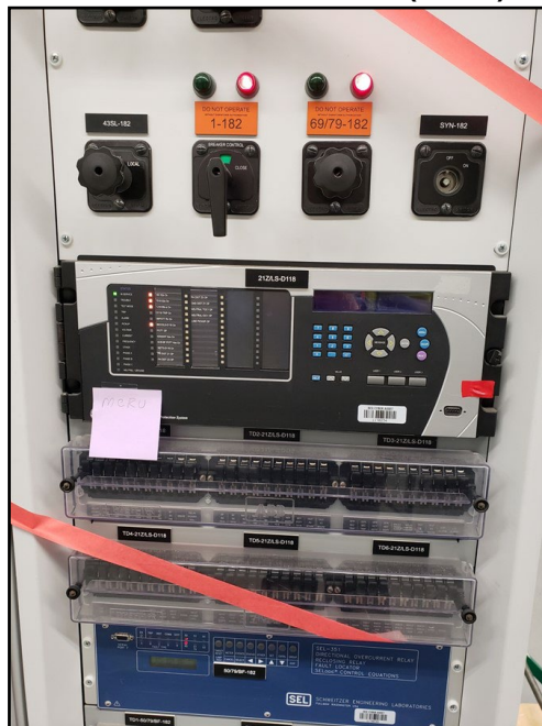
Deerfield– GE 115 kV Line D118 Secondary Protection Relay
