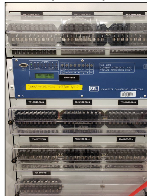
Deerfield– SEL TB14 Primary Transformer Differential Protection Relay
