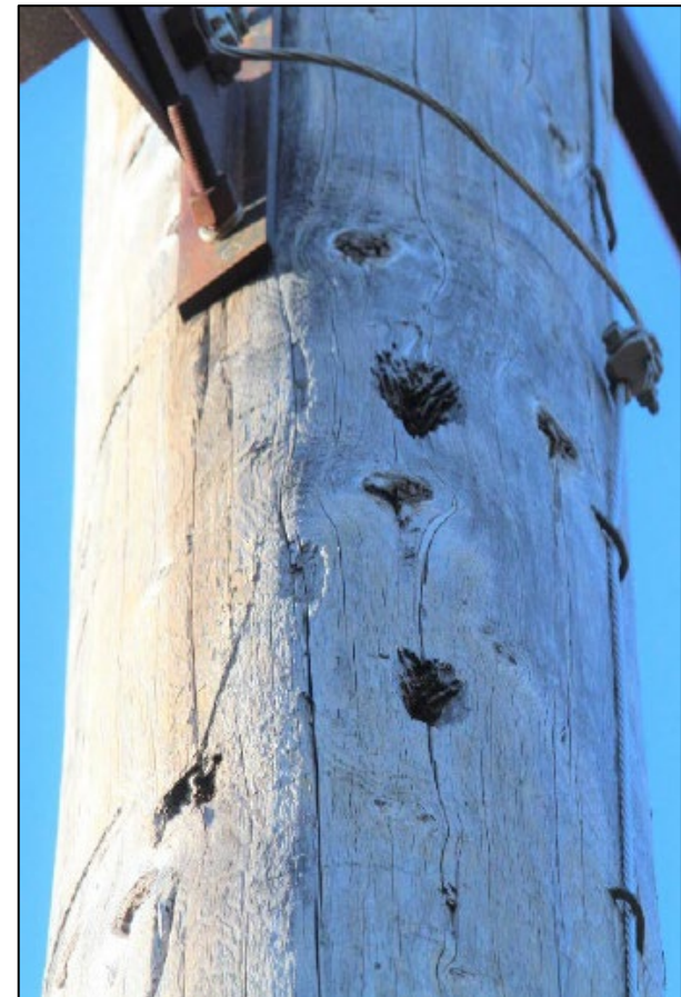
Line 364 Structure 5557 Woodpecker Damage
