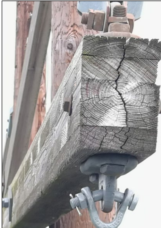
Line 1726 Structure 8084 Crossarm Cracking
