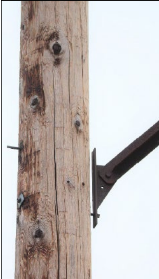
Line 364 Structure 5555 Loose Hardware
