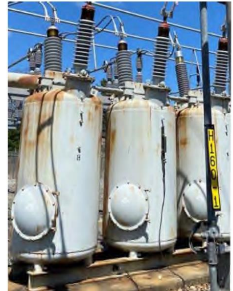
H160 115kV OCB
